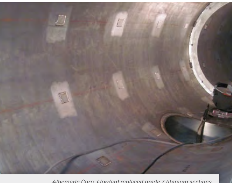
Albemarle Corp. (Jordan) replaced grade 7 titanium sections of bromine distillation columns with lower-cost, grade 2 titanium enhanced with TIMETAL PGMA patches in early 2008. The vessel has since shown no signs of corrosion.
